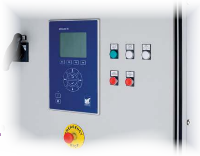
Unisab control for heat pump application
