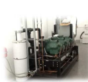
Freezer Cold Room Cyprus
