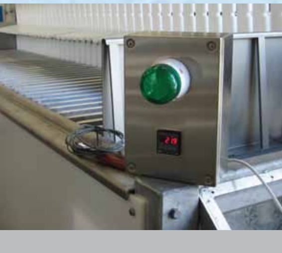
Control box for each freezer.
